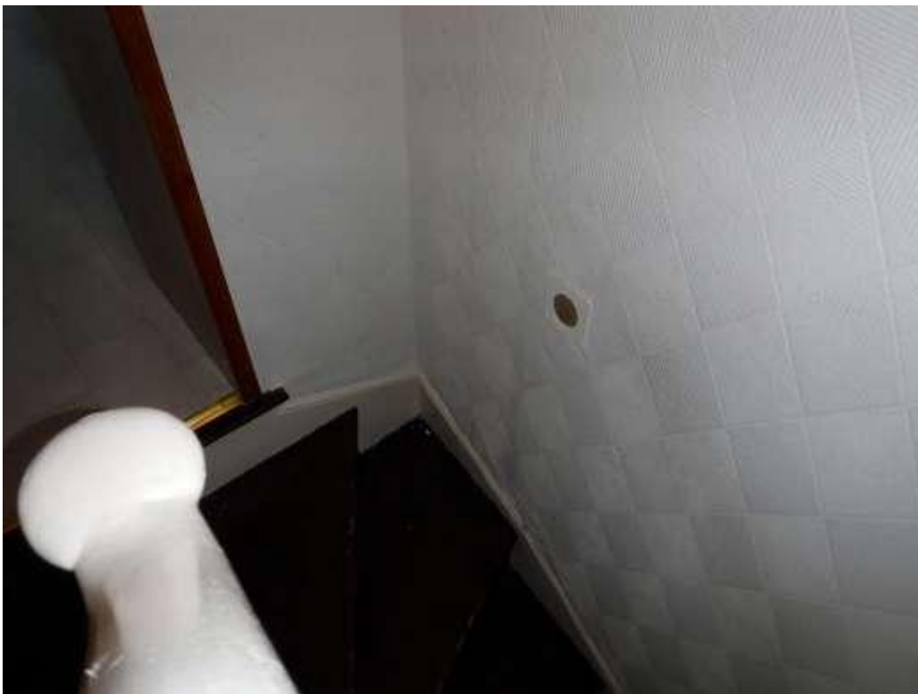
Photo 6 Damp noted at the side of the staircase.
