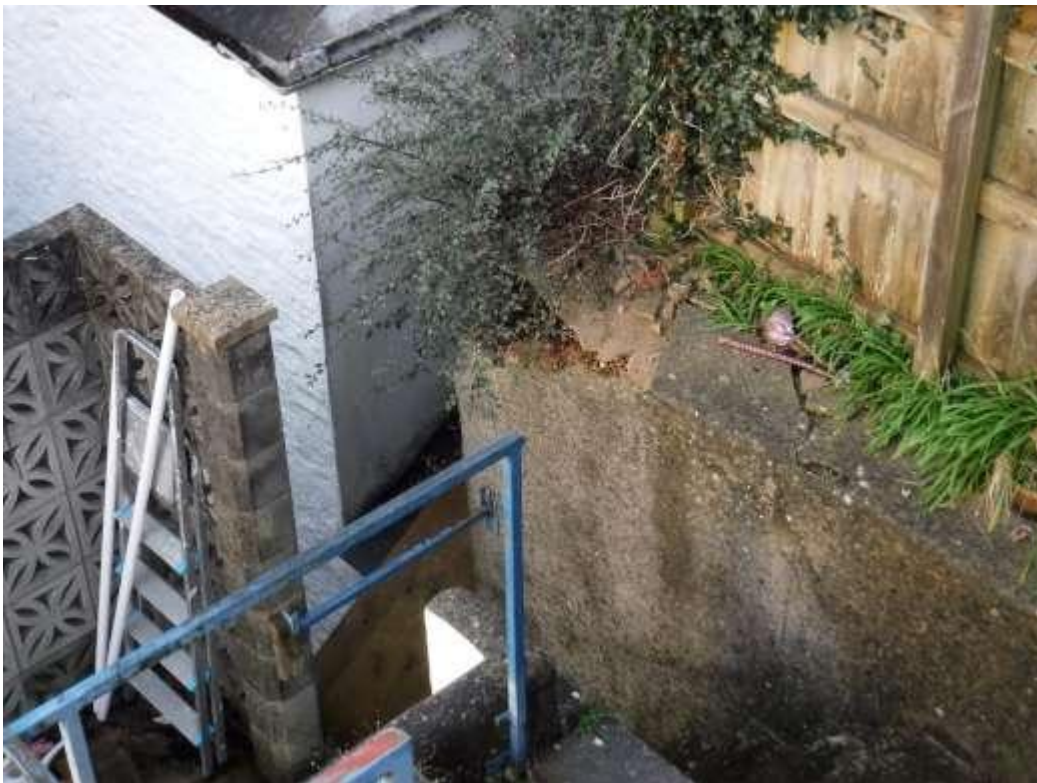
Photo 24 The retaining walls at the rear require repair.
