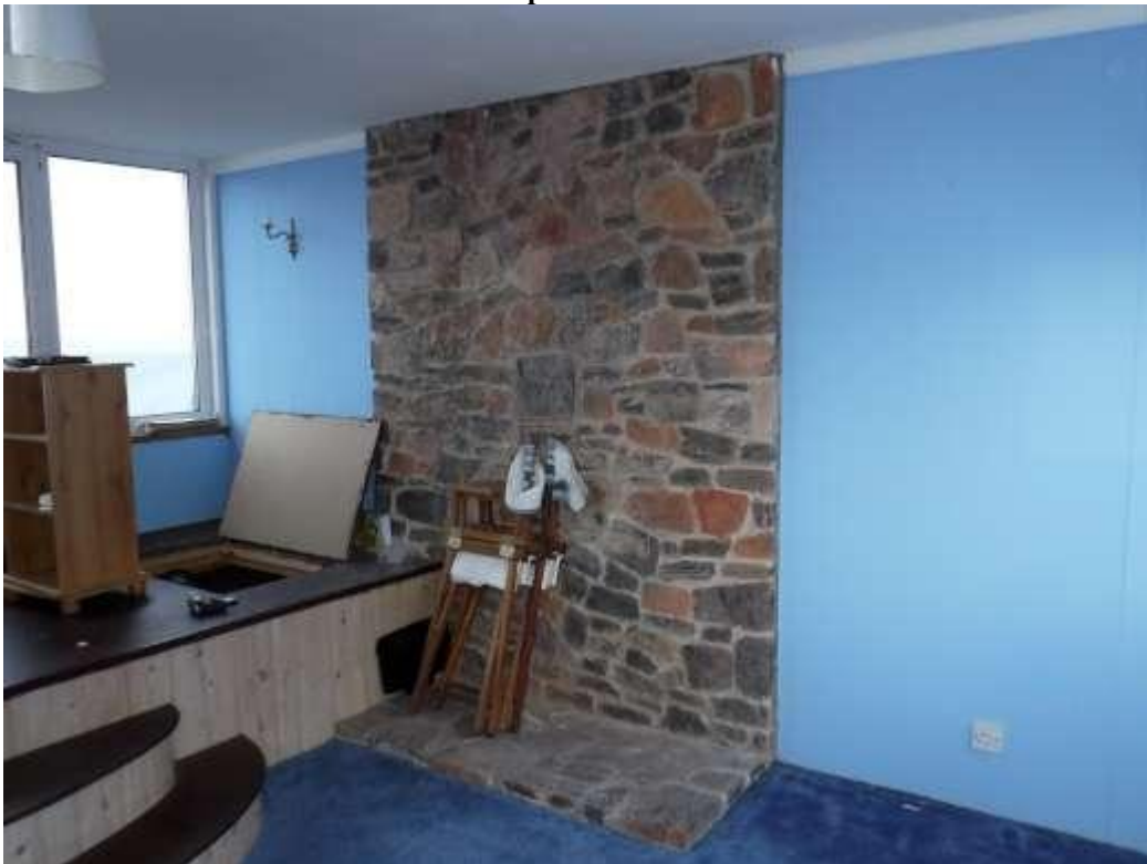
Photo 10 The hearth on this fireplace should be removed.
