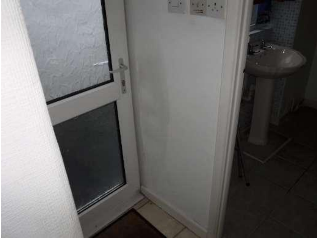
Photo 11 Rising damp noted here. Note some of this is quite high up on the wall.
