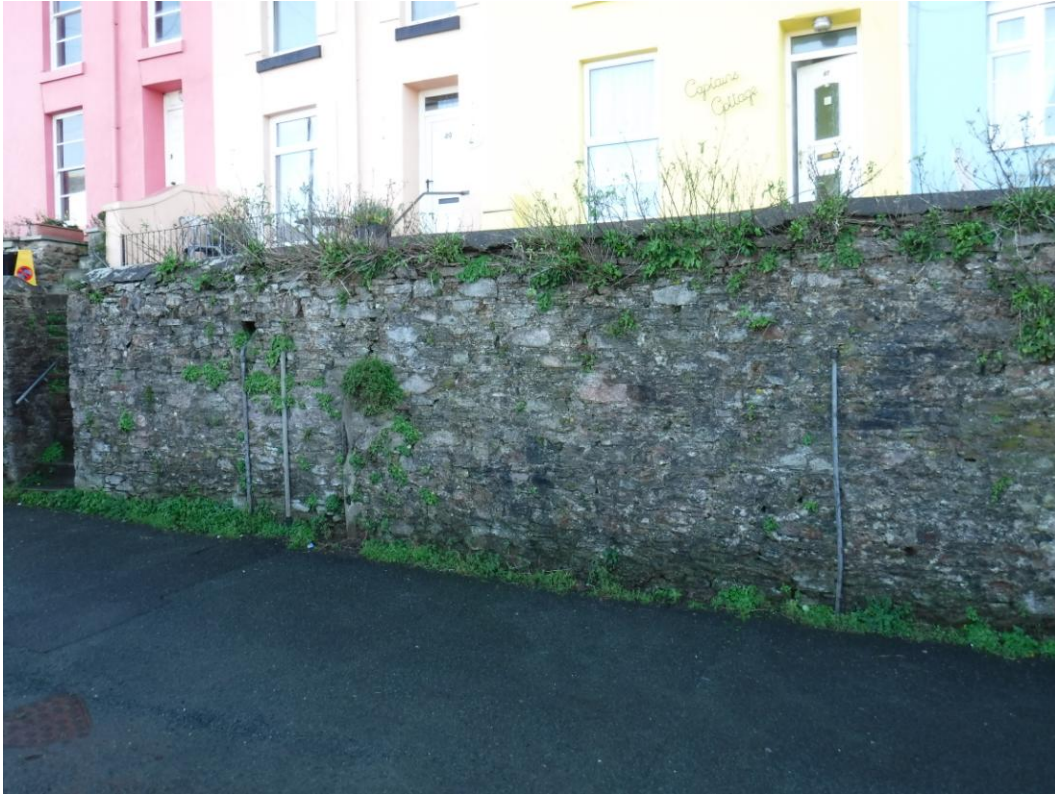
Photo 21 The retaining wall at the front requires some general maintenance.
