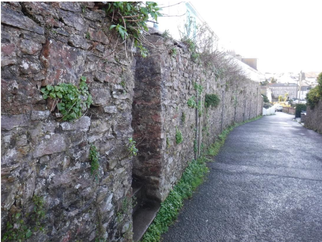
Photo 22 The retaining wall at the front requires some general maintenance.
