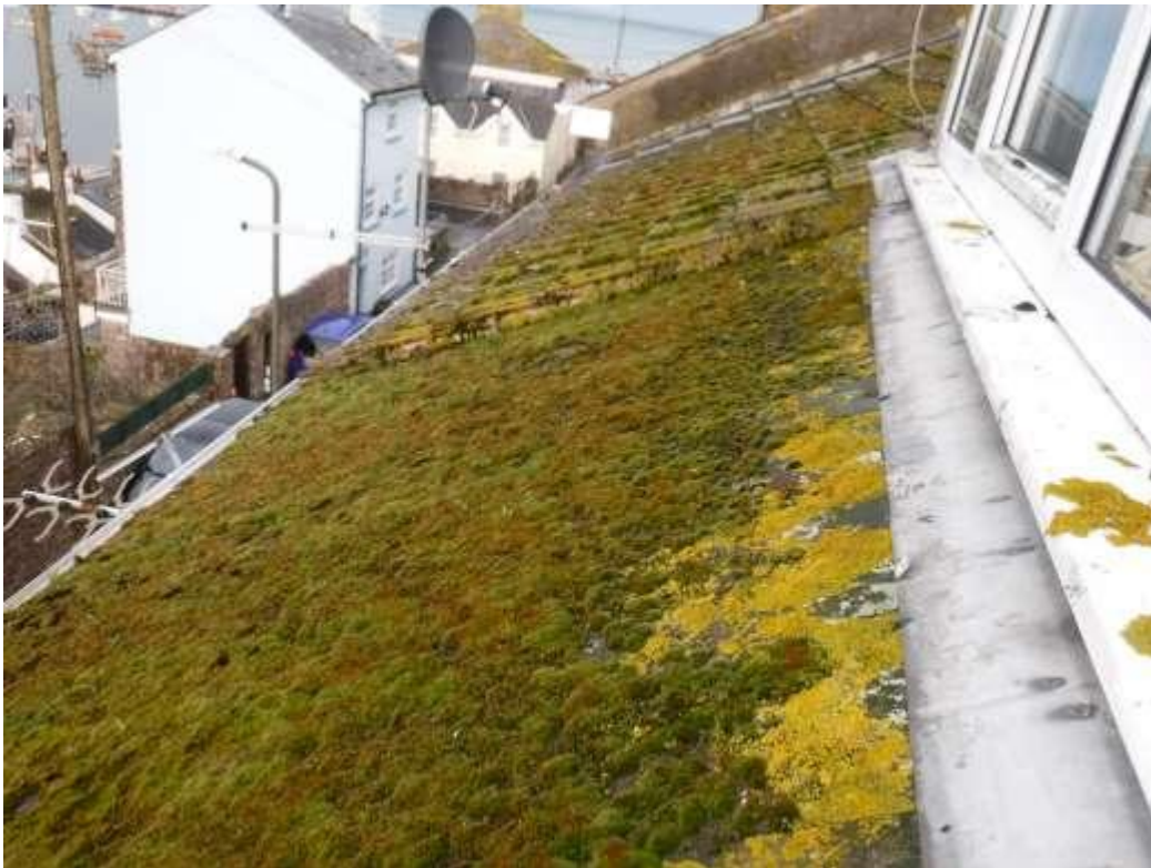
Photo 2 The left hand part of the front roof slope is in poor condition.
