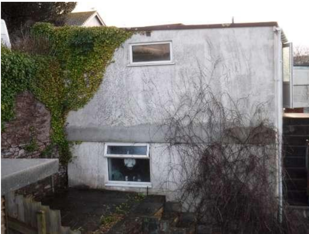
Photo 14 Right hand elevation of the out building. Note cracking above window opening and crooked window at upper level.
