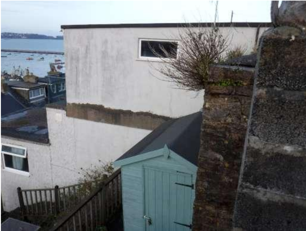
Photo 15. Left hand elevation to the outbuilding. Note repairs have been carried out to the render in the past.
