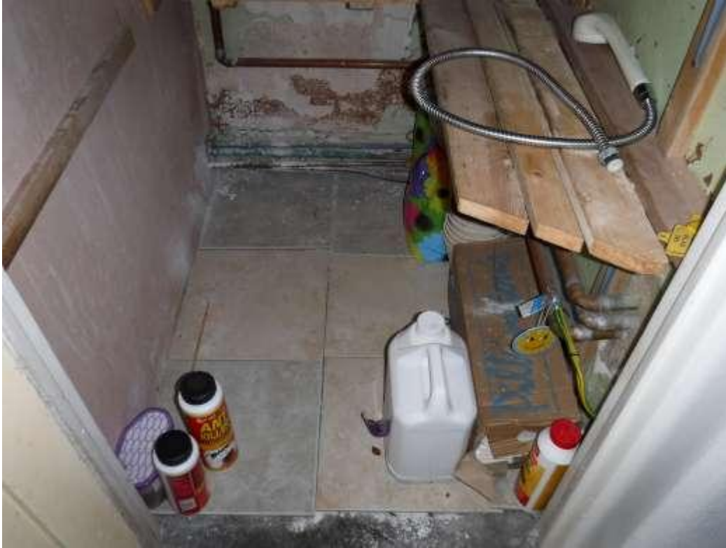
Photo 9 Damp noted in the downstairs cupboard. These floor tiles have been loosely laid and we did note some dampness underneath.
