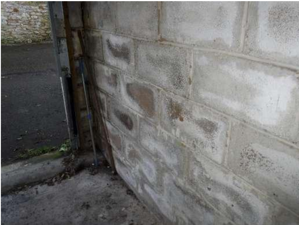
Photo 20 Dampness noted inside the garage.
