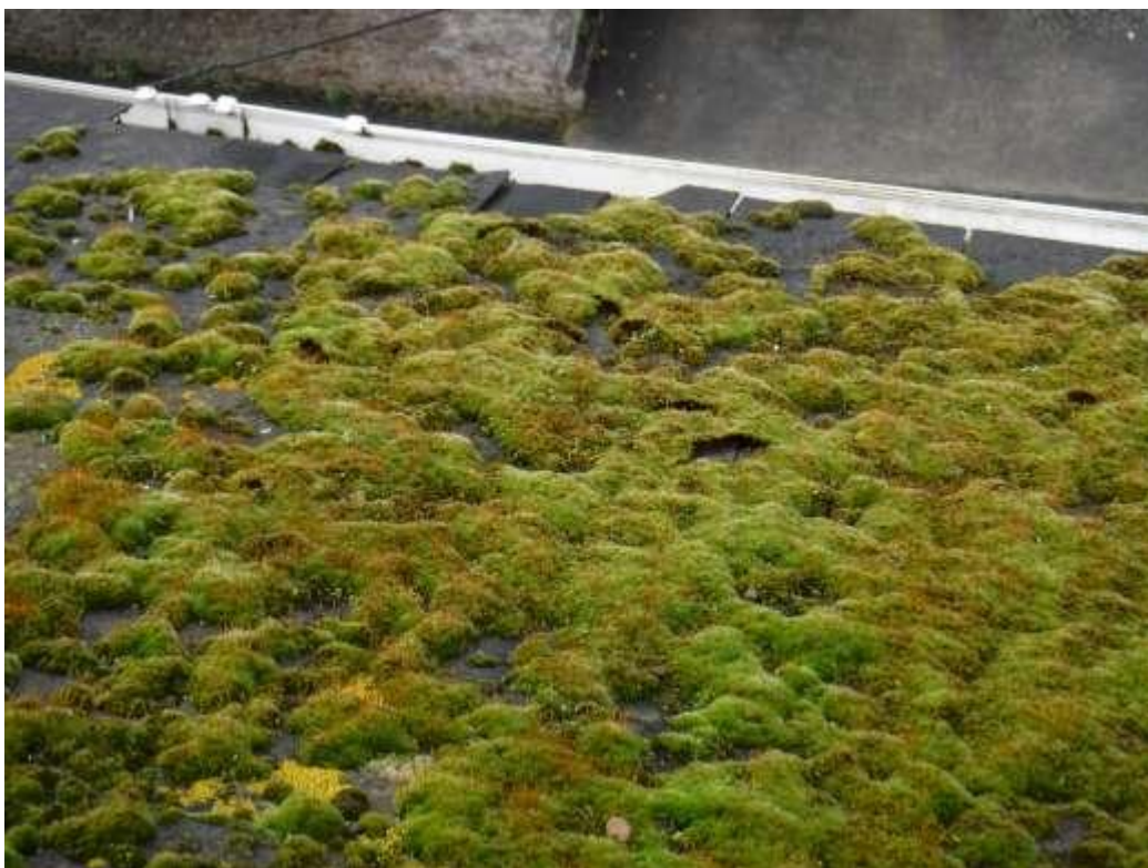
Photo 4 Some damage noted to the slates at the front.
