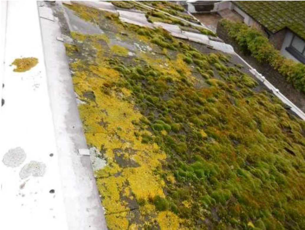
Photo 3 The right hand part of the front roof slope is in poor condition.
