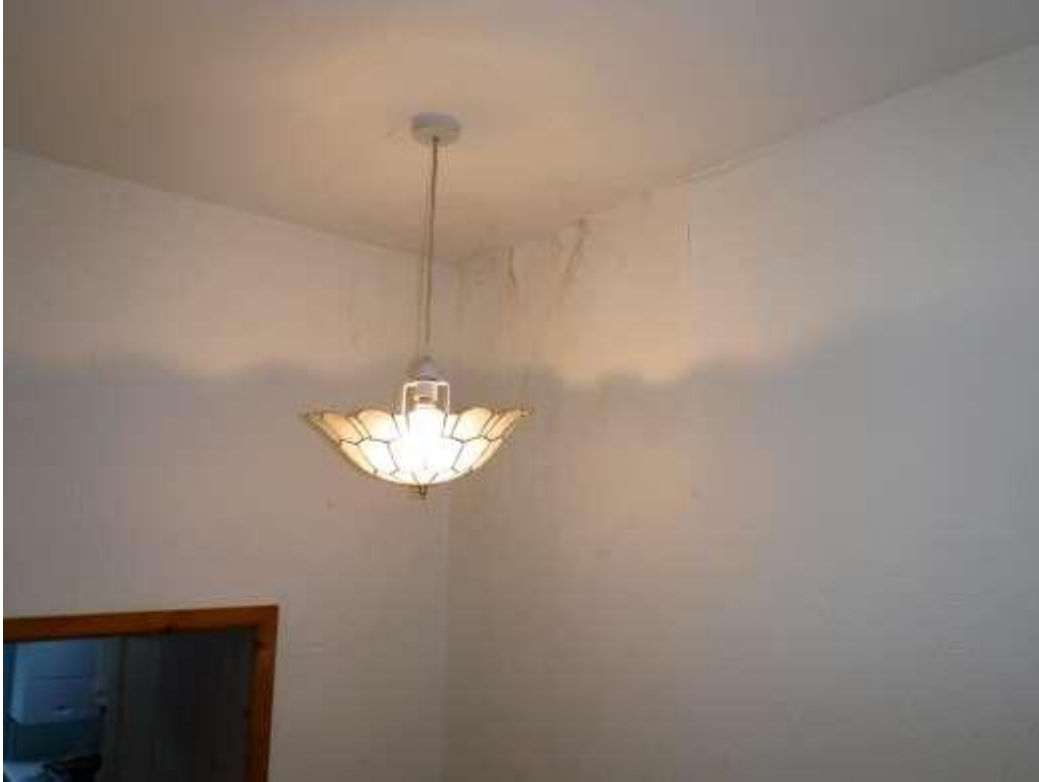
Photo 7 Damp noted at the side of the staircase.
