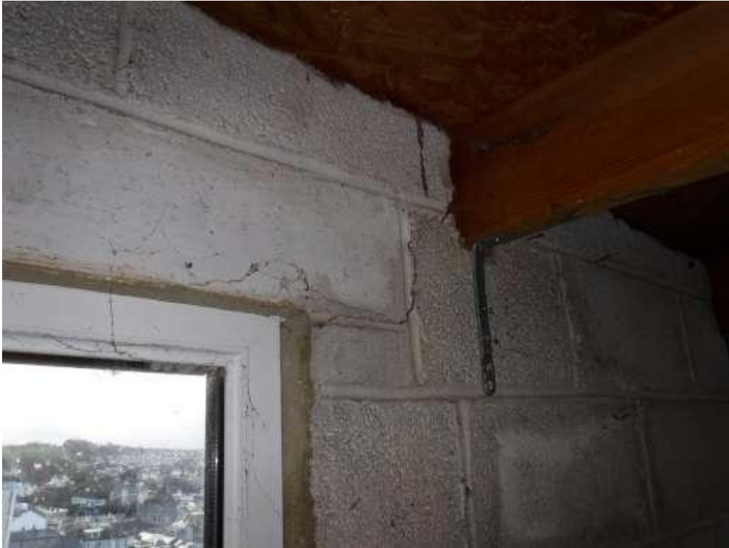
Photo 19 Movement cracks in the garage.
