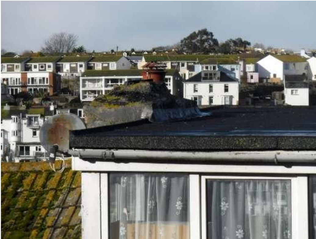
Photo 5 The right hand chimney stack requires attention.
