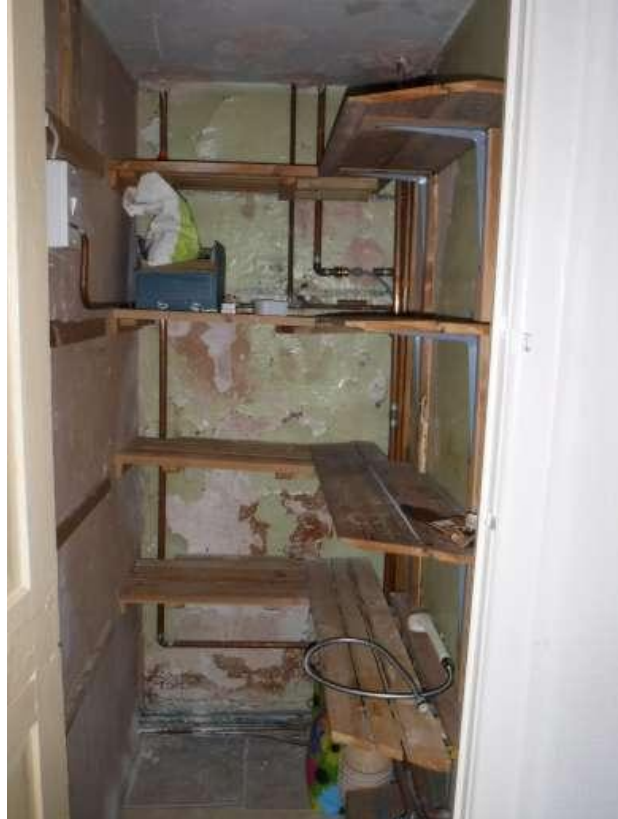
Photo 8 Damp noted in the understairs cupboard.
