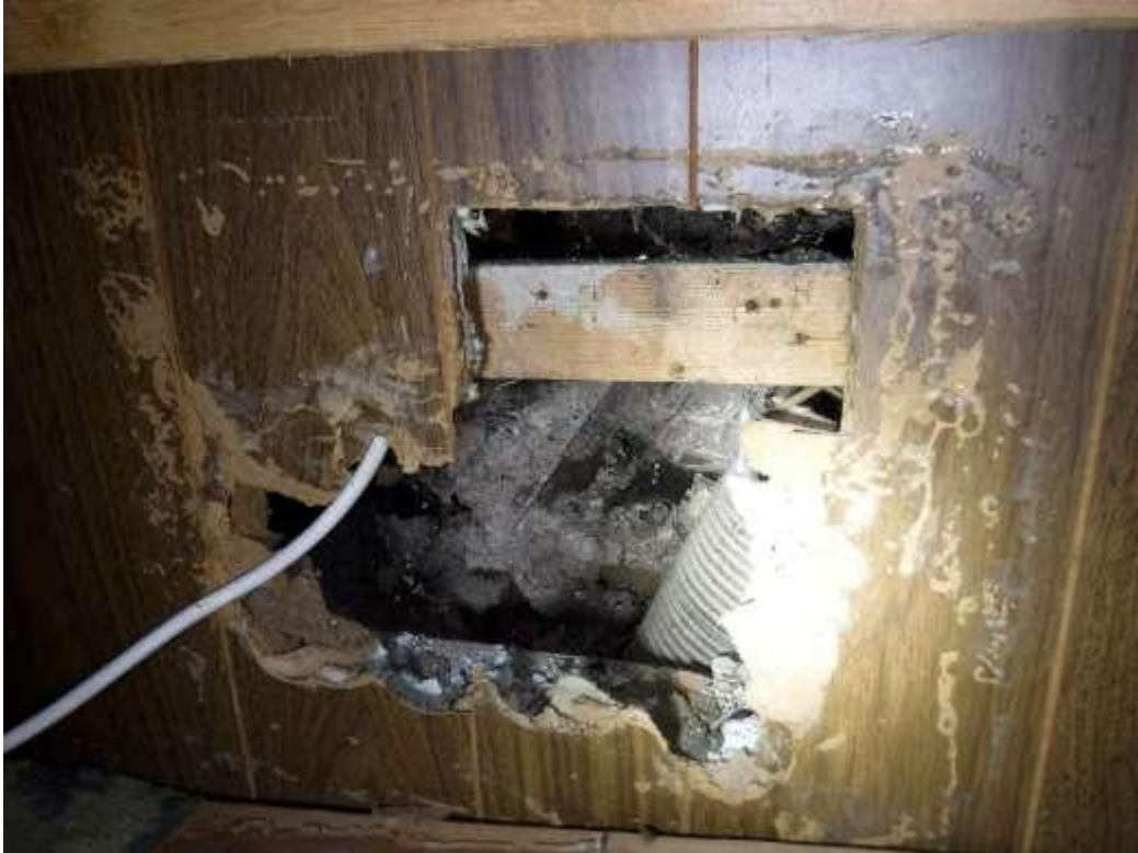
Photo 12 Where we gained access into the timber studwork around the second floor we found no vapour barrier and no insulation.
