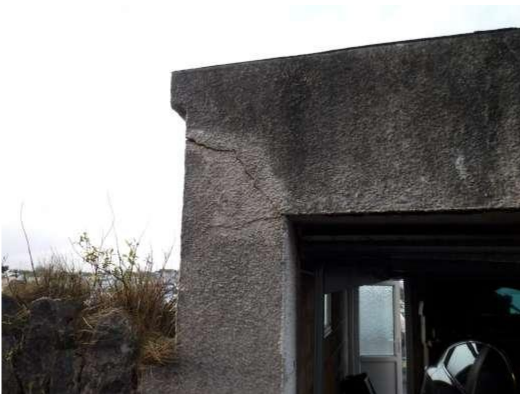
Photo 18 Movement cracks in the garage.
