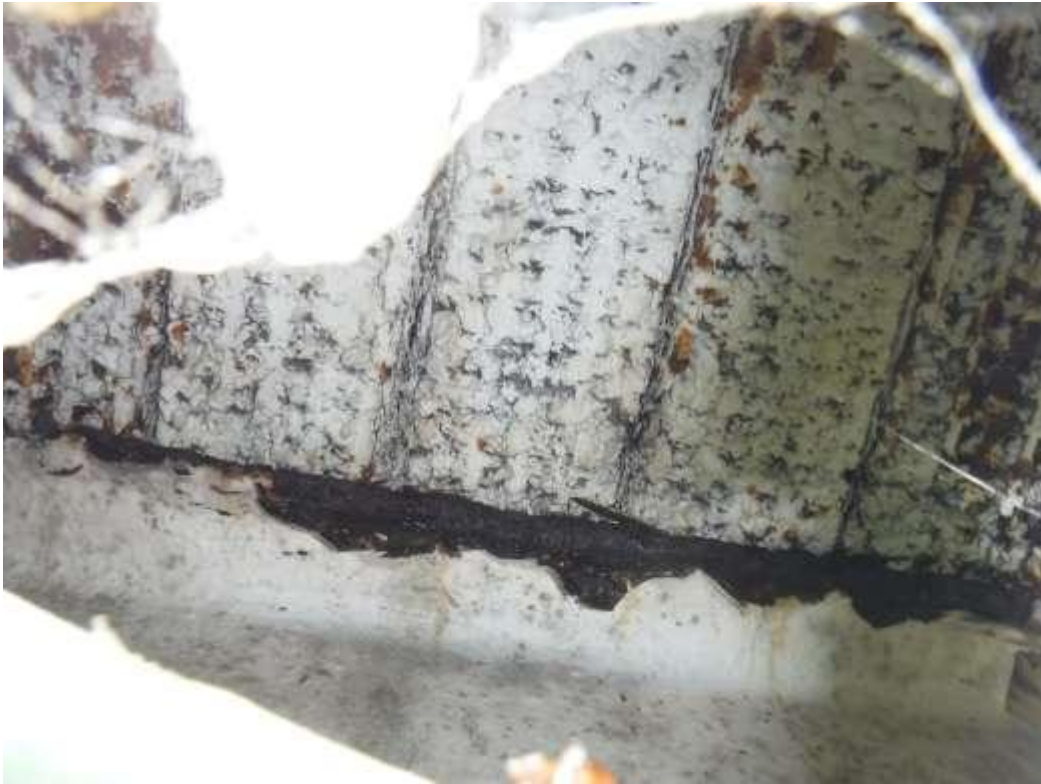
Photo 17 Corrosion and dampness noted in the concrete floor to the garage.
