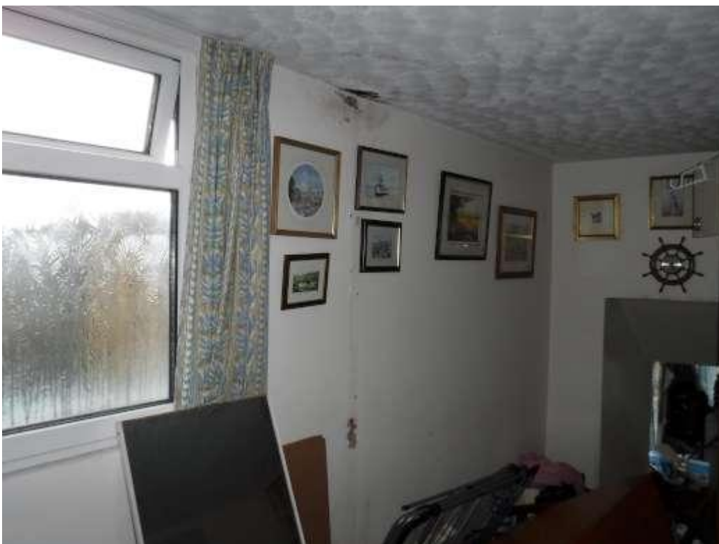
Photo 16 Damp has been getting in through the roof here.
